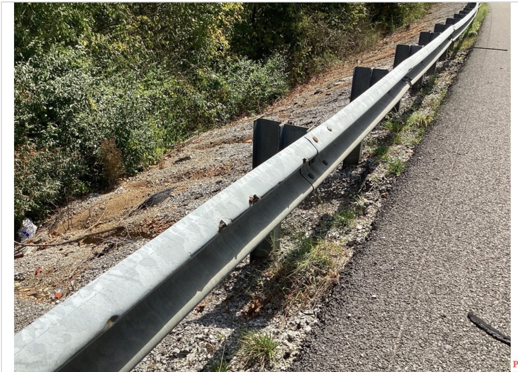
Right bridge rail - minor collision damage
