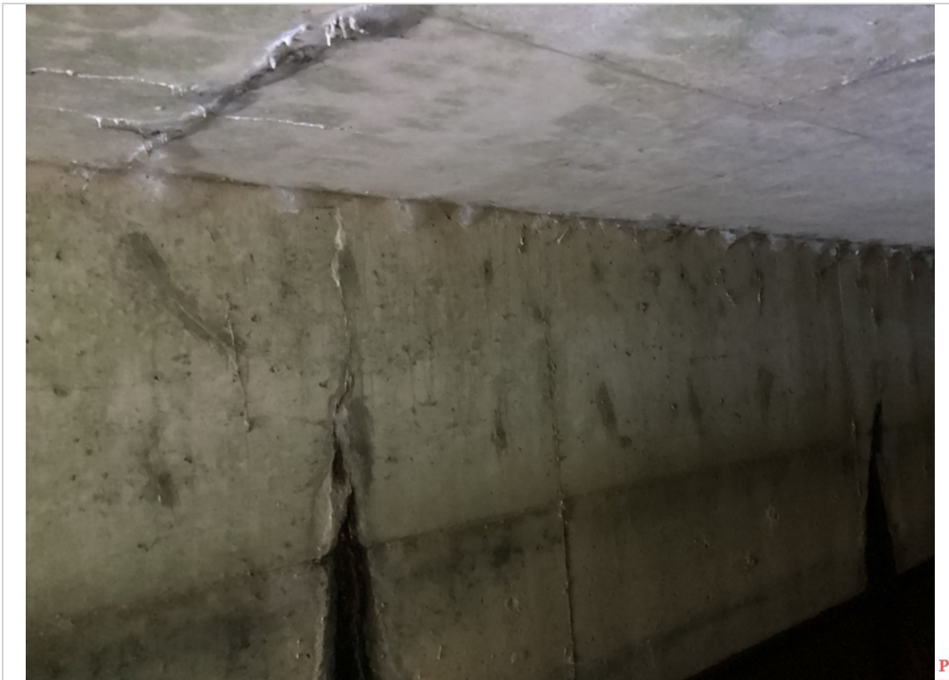
Barrel 2 - Hairline cracks w/ leaching (Typical barrel 1
