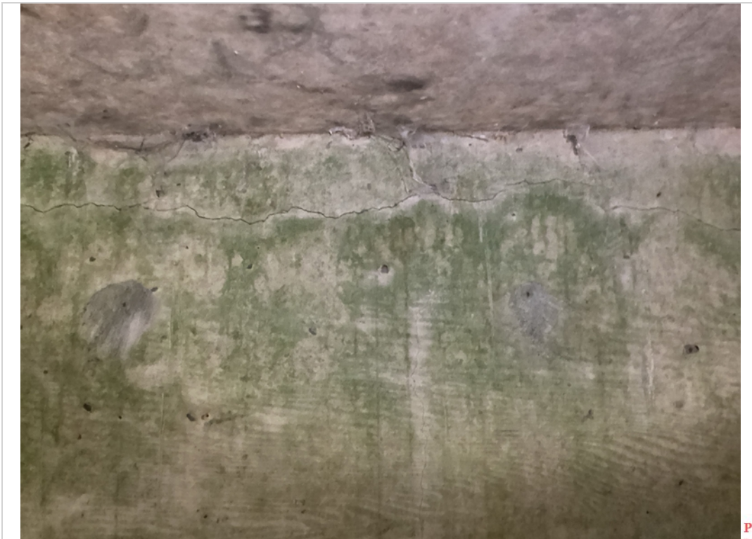
Barrel 1 wall 2 - 1/16" crack about 3" from top
