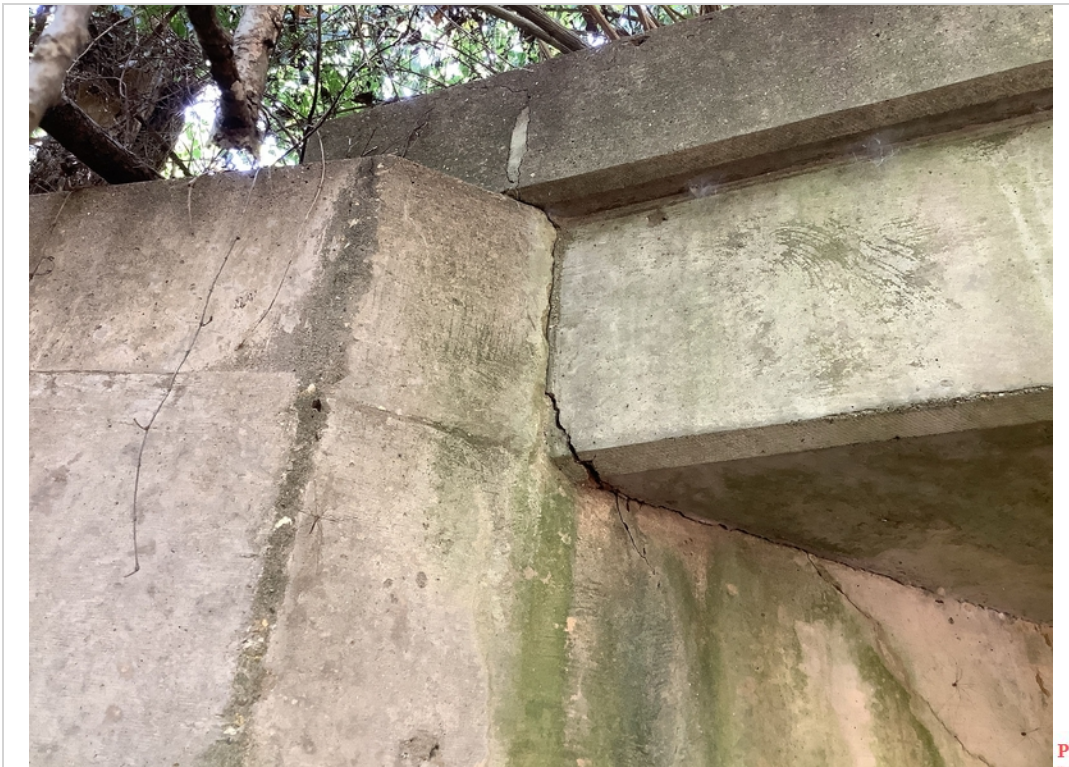
Inlet headwall at barrel 1 - cracks to 1/8"
