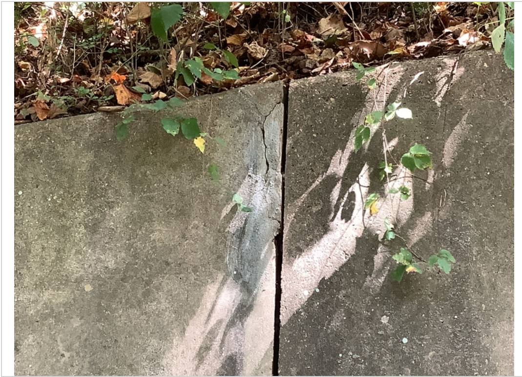
Wing 2 left - patch and spall in place (14" x 3")
