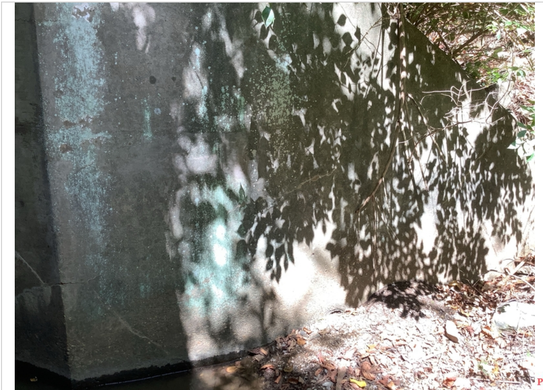
Wing 2 right - hairline cracks
