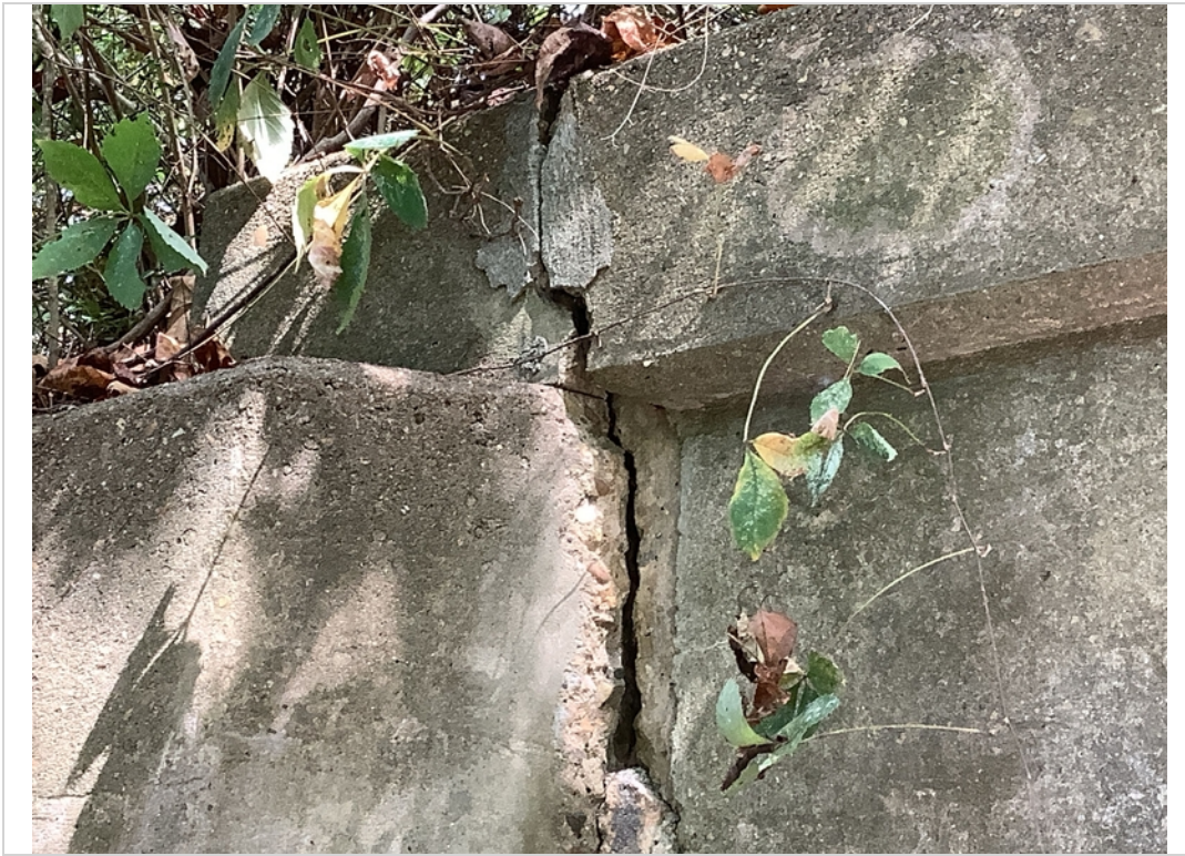
Wing 2 left abutment joint - cracks to 3/8", patch, minor spall
