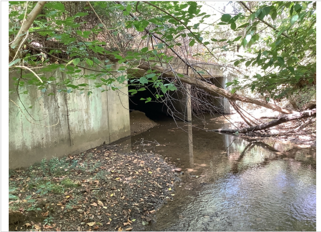
Elevation right (note fallen tree)
