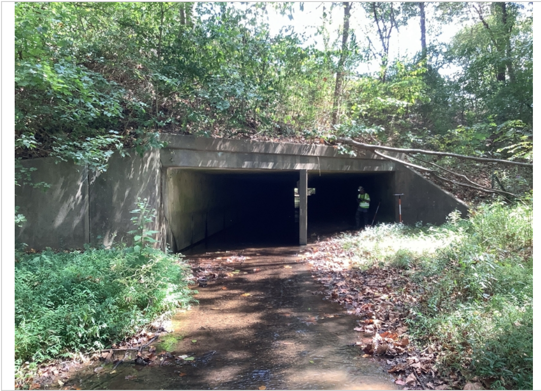
Elevation left (note fallen tree)
