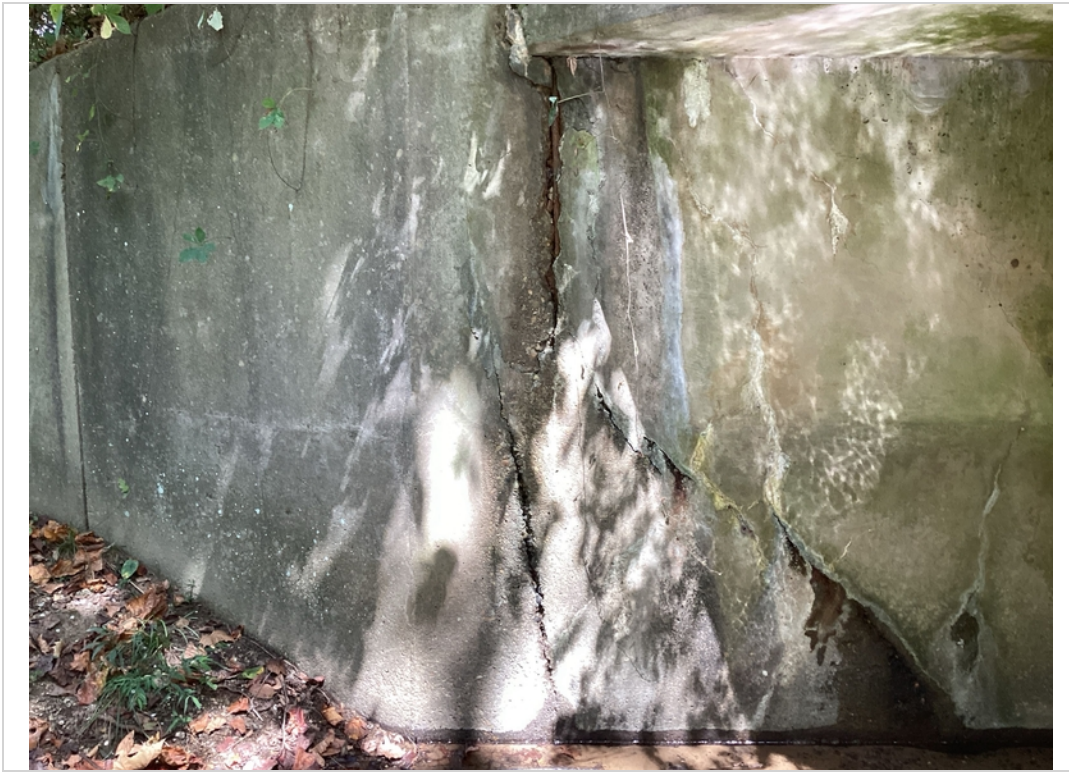
Barrel 2 left - Spall w/ exposed rebar, in place spall (3'Hx3"Wx2"D) w/ crack up to 3/8"
